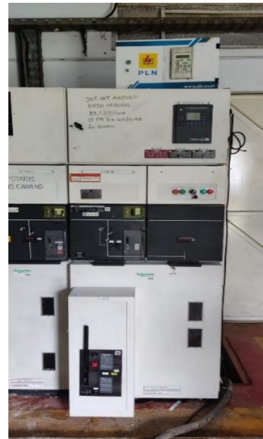
Figure 7. ACO-MV device by Talus brand at substation E20B.
