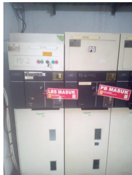
Figure 6. Cubicle at Substation E258
