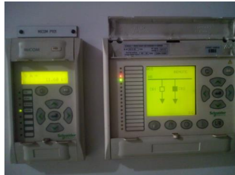
Figure 5. ACO-MV device by Schneider brand at substation E258.
