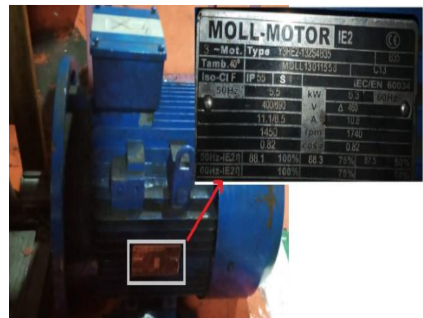
Figure 4. Induction Motor 5,5 KW
