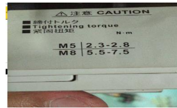
Figure 2. Example of Standard Bolt Tightness on MCB 25 Ampere
